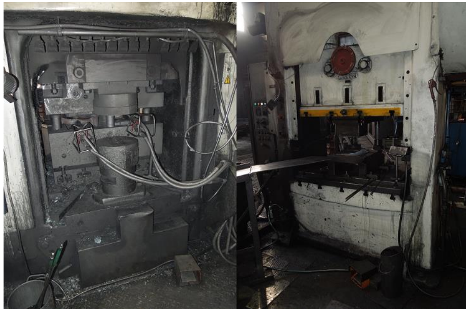
Figure 17 – Clamped tools on forging press (left) & trimming press (right) (own processing)
