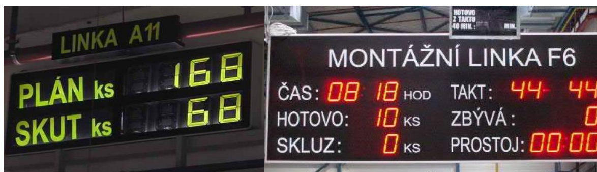
Obr. 71. Monitorovací systém – LED panely (RTG-TENGLER, ©2015)
